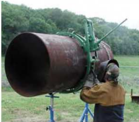
Hydraulic Cage Clamps permit rapid pipe alignment and quick release of the clamp from the pipe after welding.
