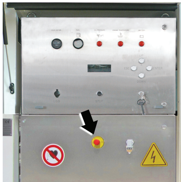
a. Command and control panel
